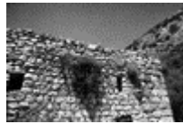
23 Iscandria flour mill (?) at Nahal Ammud River near Safed. The Middle East, April 19, 2001
