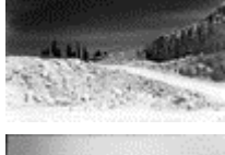
30 A road under construction through chalk stone 2 miles north-east from BGU. Beer-Sheva, the Middle East, May 12, 2000
